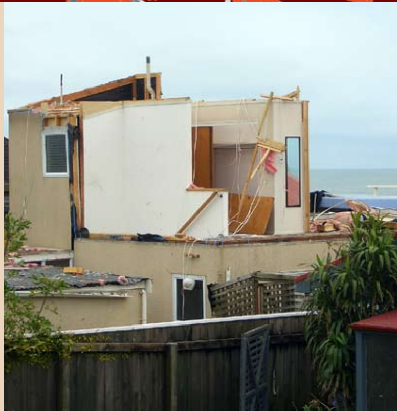
Smashed – a house in Oakura after the tornadoes struck. [Photo: Peter Scantlebury, New Plymouth District Council]
